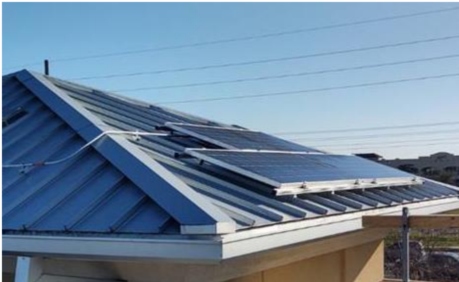
Sample photo of a completed JP Morgan Chase solar project
